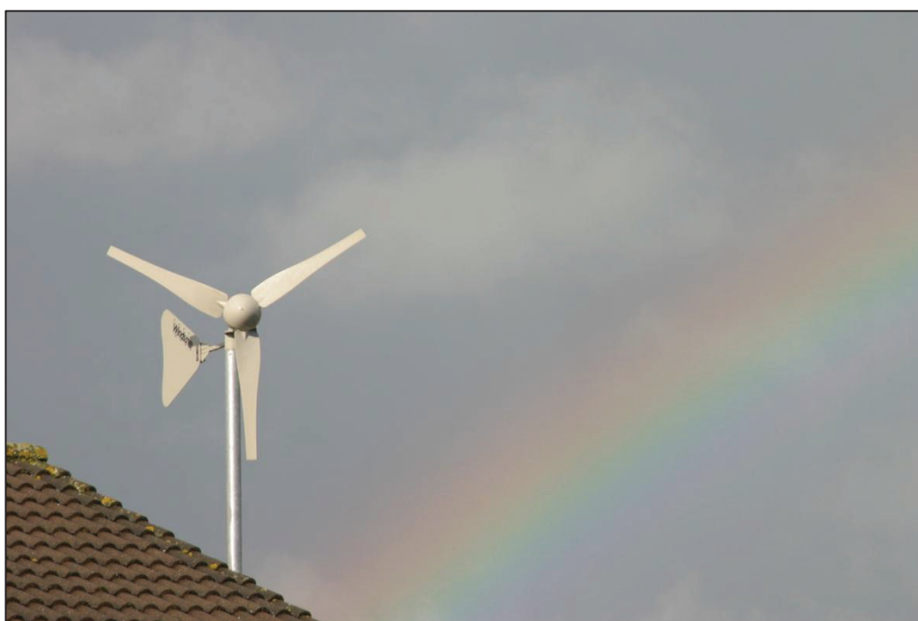
Small Wind Turbine mounted on a roof
