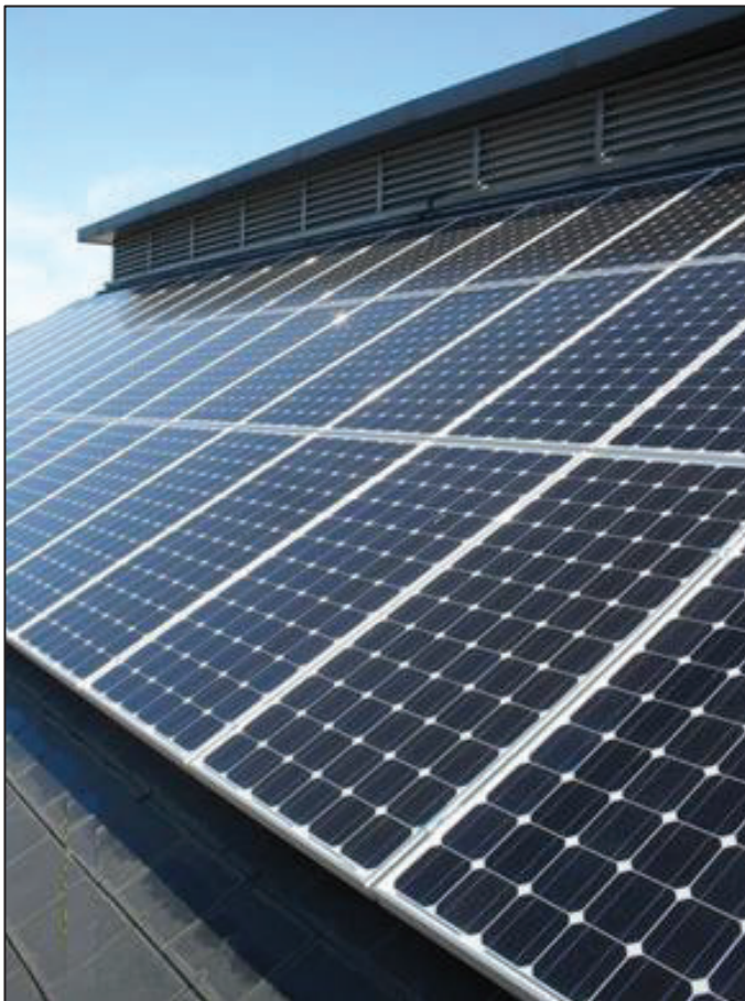
Solar panels mounted on a roof
